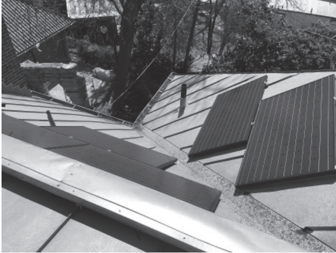
A view from the roof of the solar panels at 218 Washington St.
