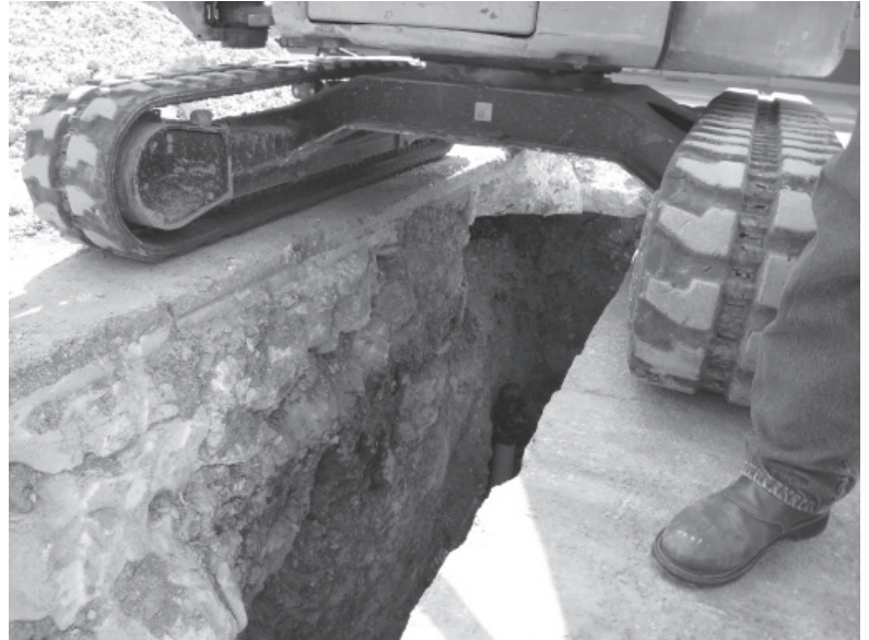
The wall of the acequia can be seen on the left, under the backhoe.
