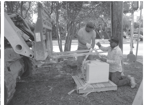
The heavy blocks are put in place with skilled hands and a backhoe.
