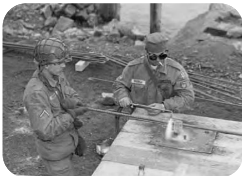
Soldiers of the 561st Port Construction Engineer Company bending rebar for a construction project. (photo circa 1960)
