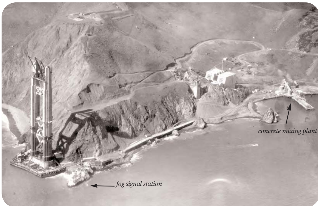
The Golden Gate Bridge was constructed between 1933 and 1937; the pier for the north tower abutted at the base of Lime Point. The Horseshoe Cove area was used as a staging area for construction activity. Note the fog signal station at the lower left and the bridge-related concrete mixing plant just north of the Needles. (photo circa 1934; courtesy of the Golden Gate Bridge District)
